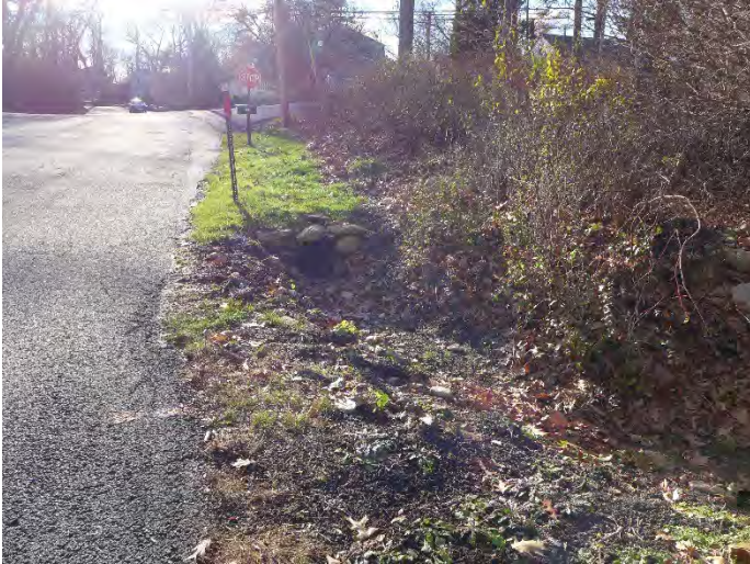
Photo 7: Sheet flow condition at pavement edge
