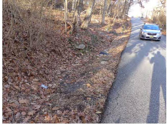
Photo 14: Pleasant Road existing ditch with bare soil; looking north.
