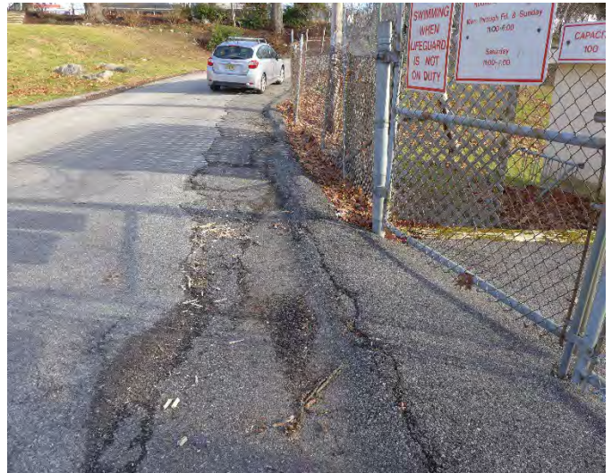
Photo 98: Curbed portion of Point Drive and paved drive at gated entry; no storm inlets.
