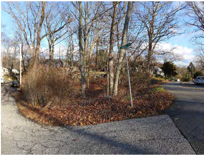
Photo 5: Sheet flow condition at pavement edge
