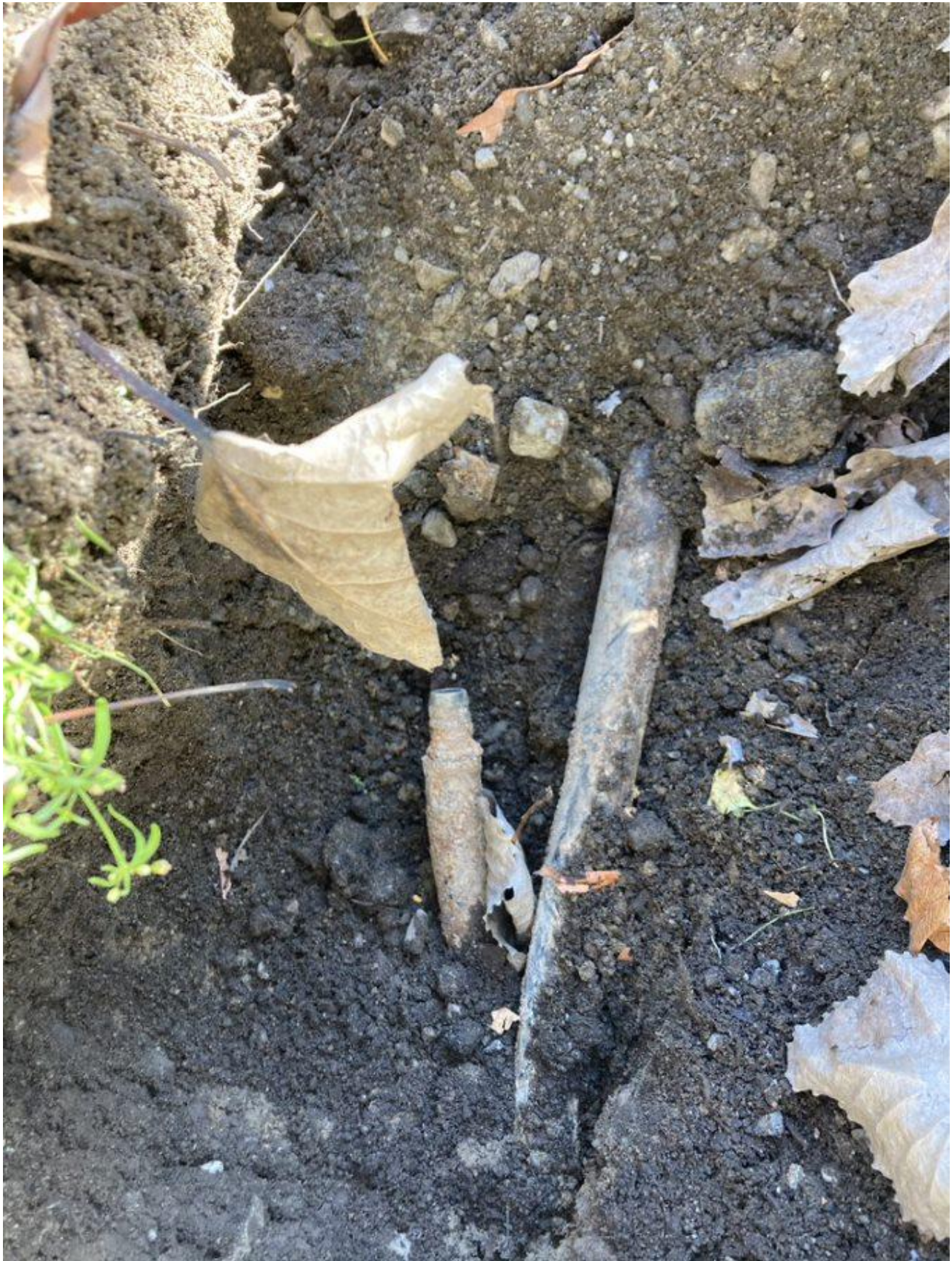
Image 2: The break in the airline to the deepest diffuser was discovered and repaired.
