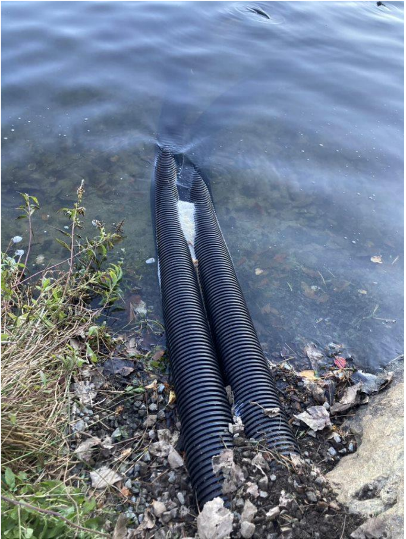
Image 3: New airline between the shed and waterline was enclosed with corrugated UV-resistant pipe
