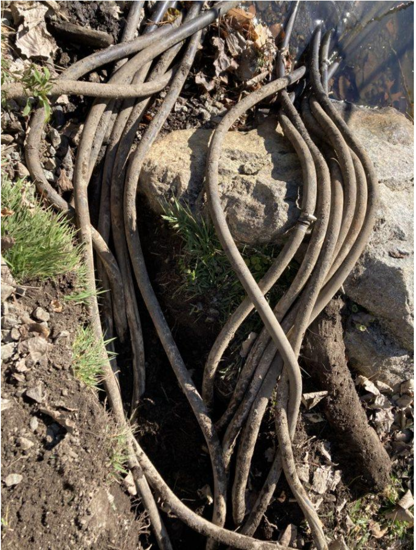
Image 1: Airlines between the shed and the shoreline were excavated to locate break in airline to deepest diffuser. Airlines for all diffusers were replaced in this section with high-temperature airline.
