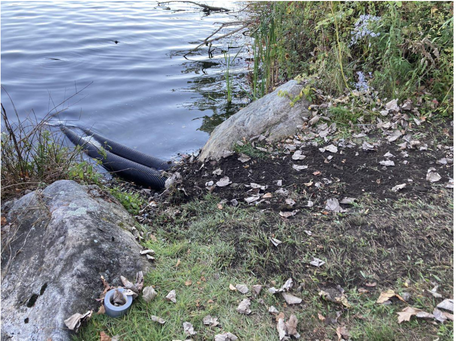
Image 4: Overview of repairs, with corrugated pipe buried and extending into lake. The pipe extends approximately 10 feet into the lake, as does the new, high-temp airline. This will protect the airline from degradation by UV rays and reduce the likelihood of splits or ruptures.
